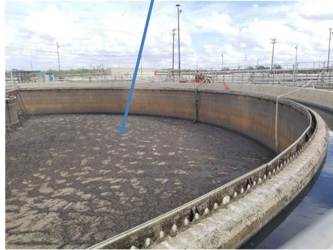
10 REMAINING SLUDGE AT BOTTOM OF CLARIFIER SCALE: N.T.S.
