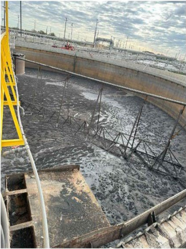
9 REMAINING SLUDGE AT BOTTOM OF CLARIFIER SCALE: N.T.S.
